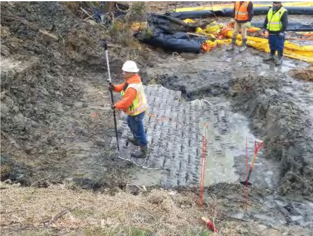
Fig 2: Installing blocks over cable at toe of slope, Gundalow landing/east side of the Bay. Viewing south. (04-30-20).
