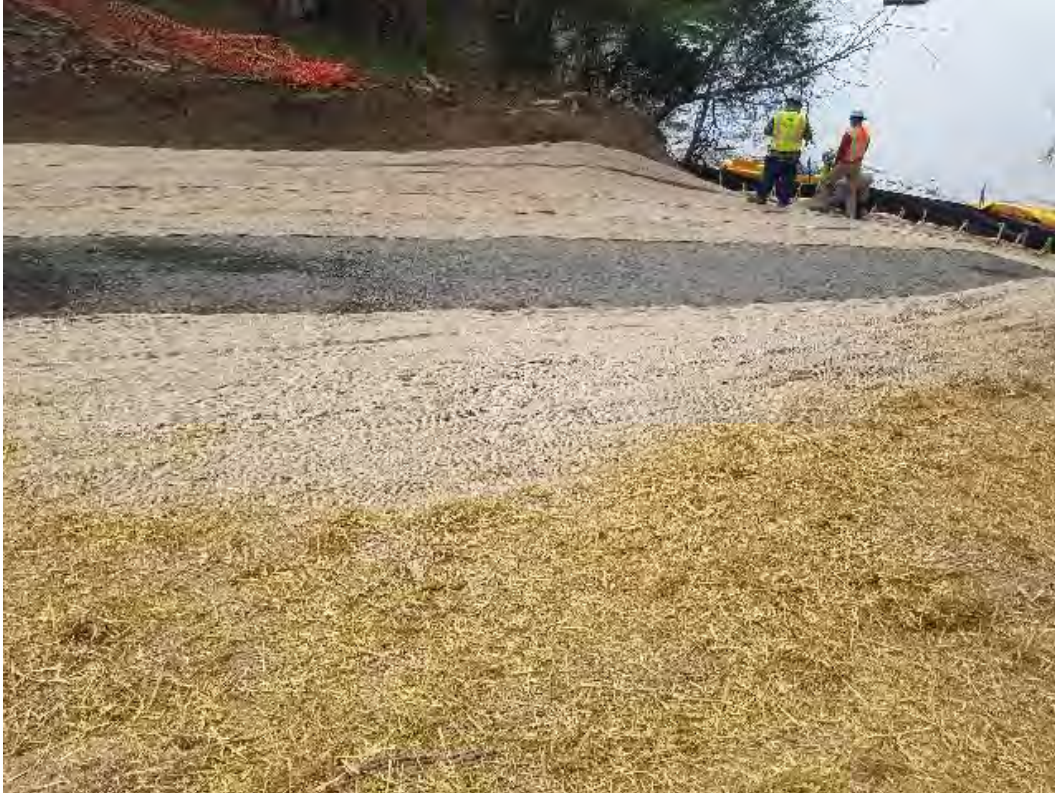
Fig 13: Seeding, installing jute mat and mulching slopes at Gundalow landing/east side of the Bay. Viewing southwest. (05-05-20).
