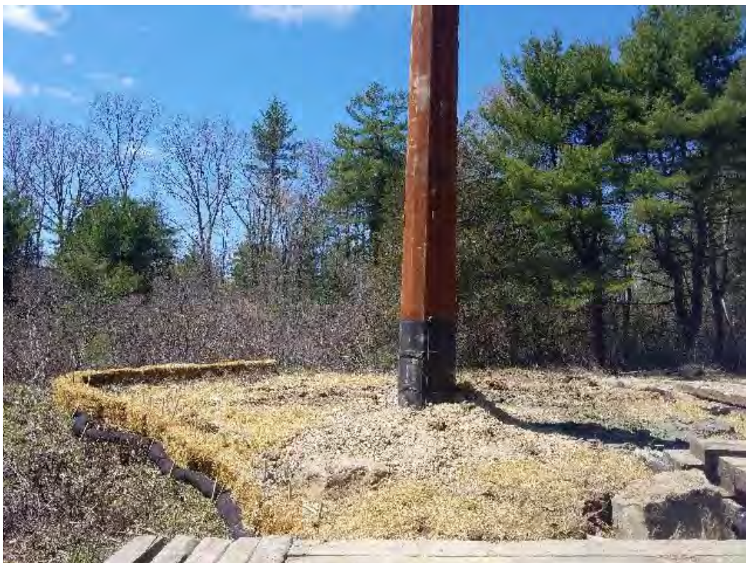
Fig 16: Str. 44 pole set. Viewing west. (05-05-20).
