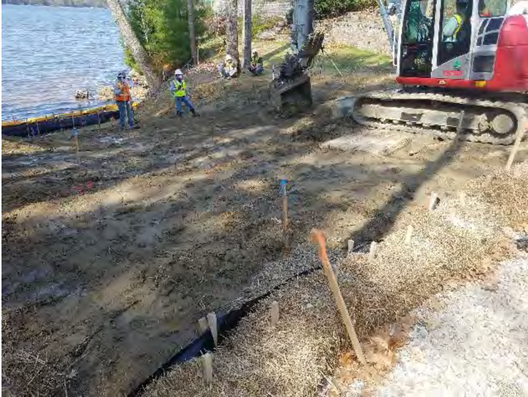
Fig 7: Establishing final slope/grade at Gundalow landing/east side of the Bay. Viewing west. (05-03-20).
