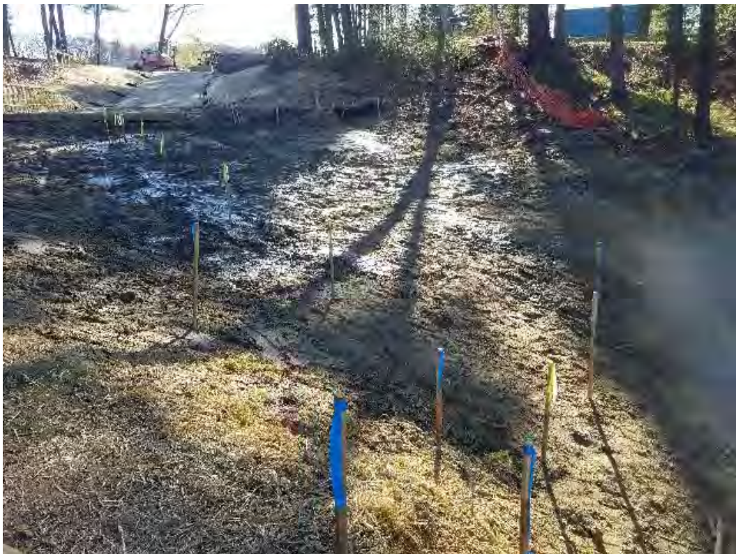
Fig 8: Establishing final slope/grade at Gundalow landing/east side of the Bay. Viewing east. (05-04-20).
