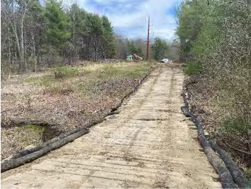
Fig 21: Access road swept and maintained over stream DS30 in wetland DW32. Between Strs. 84-85. Viewing east. (05-06-20).
