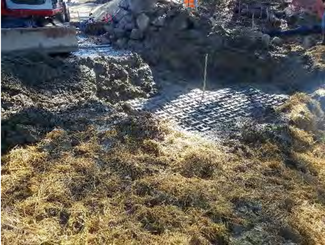
Fig 5: Installing blocks over cable at toe of slope, Gundalow landing/east side of the Bay. Viewing southeast. (05-02-20).
