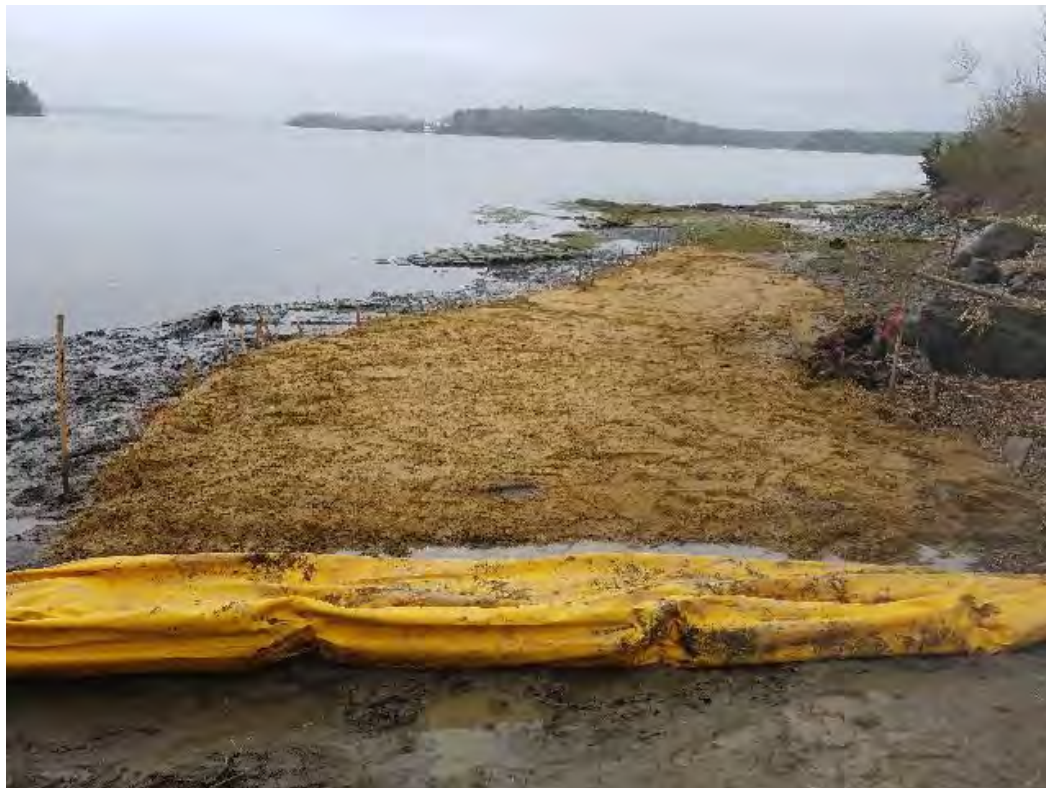
Fig 4: Material spread for base of salt marsh restoration on east side of Bay. Viewing west. (04-30-20).
