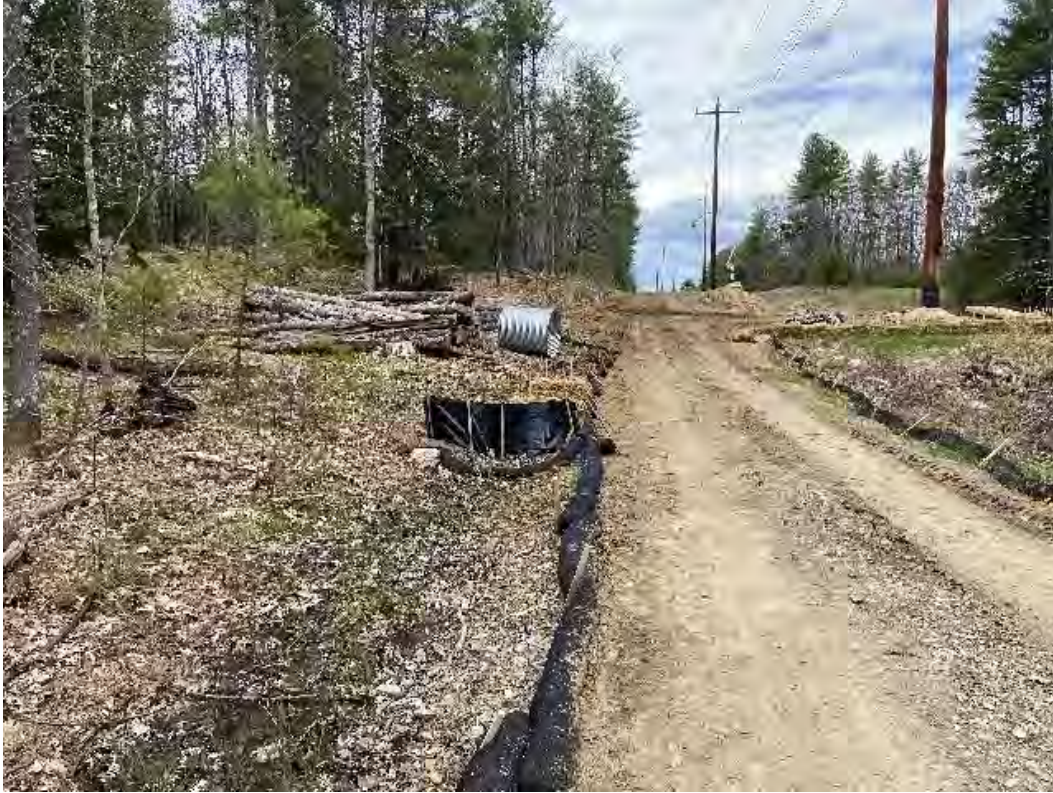
Fig 23: Silt fence installed in swale along access road to Str. 93. Viewing northwest. (05-06-20).
