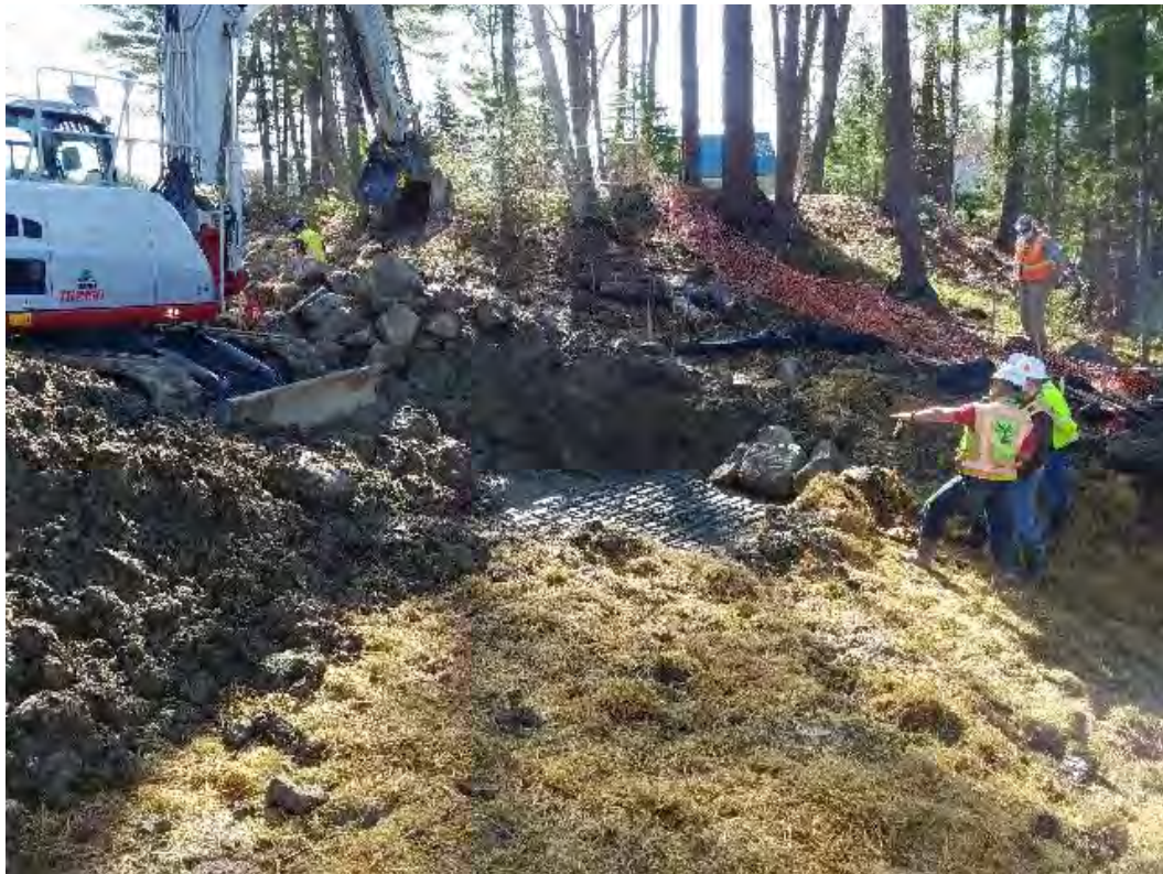
Fig 6: Backfilling over blocks at Gundalow landing/east side of the Bay. Viewing south. (05-02-20).
