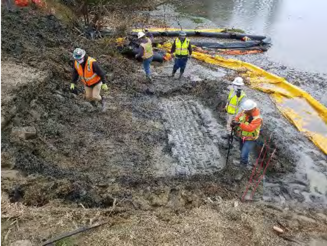
Fig 1: Installing blocks over cable at toe of slope, Gundalow landing/east side of the Bay. Viewing south. (04-30-20).
