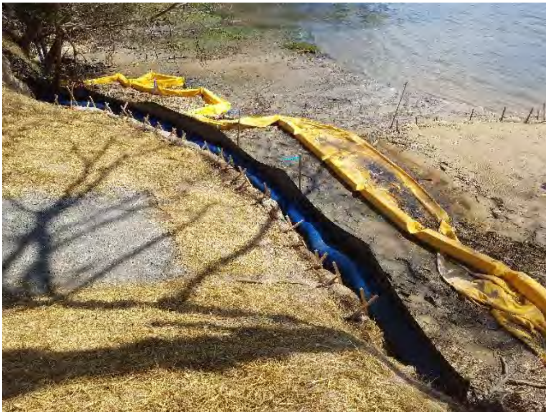
Fig 14: Installing BMPs at toe of slope at Gundalow landing/east side of the Bay. Viewing south. (05-05-20).
