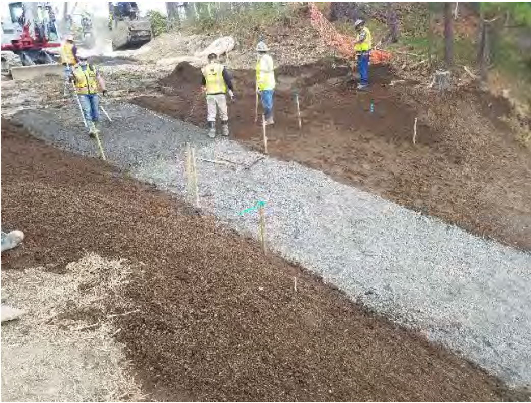
Fig 11: Spreading loam and gravel for walkway on slope at Gundalow landing/east side of the Bay. Viewing southeast. (05-04-20).
